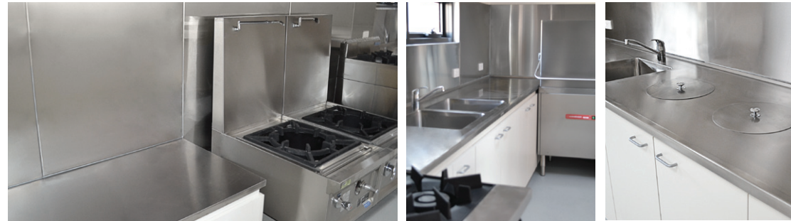
(L-R) Stainless Steel Wall Panel with Fire Rated Wall Cladding, Commercial Kitchen Sink and Dishwasher Bench, Custom Stainless Steel Bench Top with integral double bin chute and lids.
